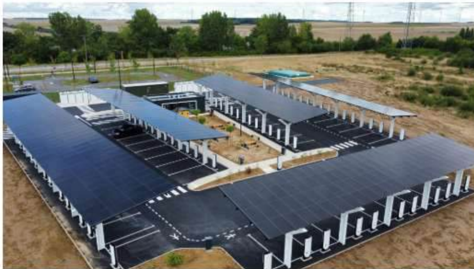
TESLA SUPERCHARGERS WITH SOLAR CARPORTS
