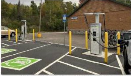
Culvers Rhinelander WI: (2) PL2.0 @ 160KW each
